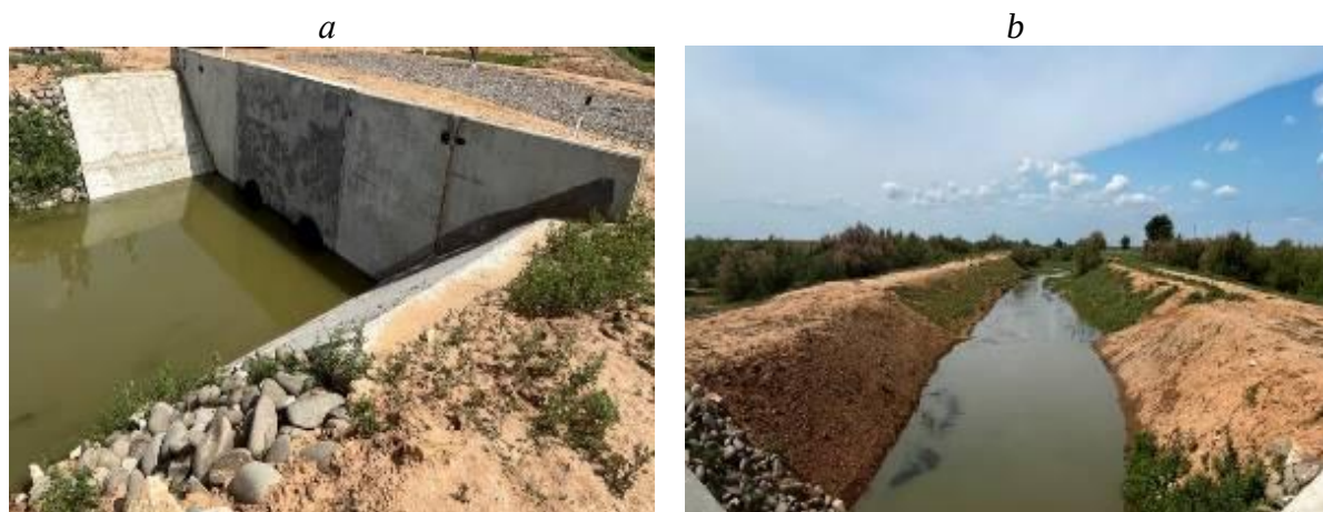
a – нижний бьеф; b – заиление и зарастание русла a – downstream; b – siltation and overgrowth of the canal bed
